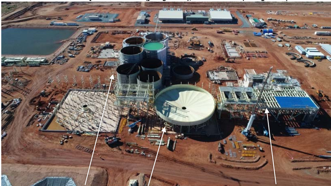
Aerial view of CIL tanks, pre-leach thickener and base structure for the SAG and Ball Mills
